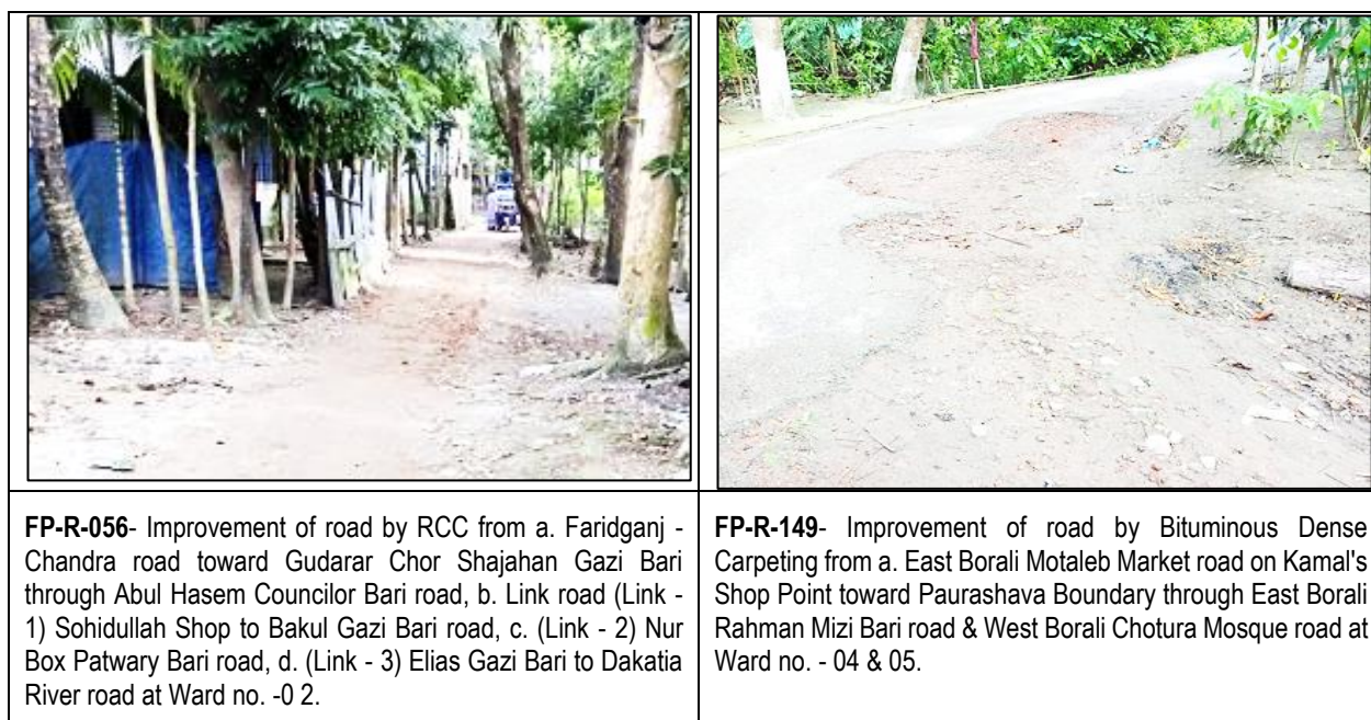
Figure 5: Existing Status of Pourashava Road
